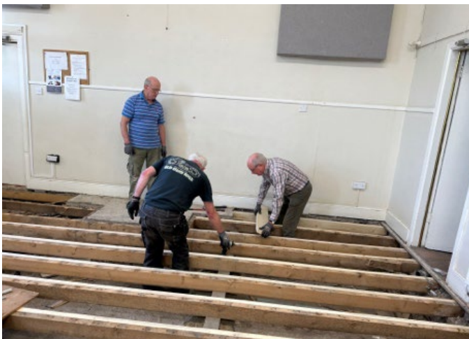
The Stripped Out Floor and Joist Re enforcement by Brendan Howley, Michael Bolger and Dan Leo.
