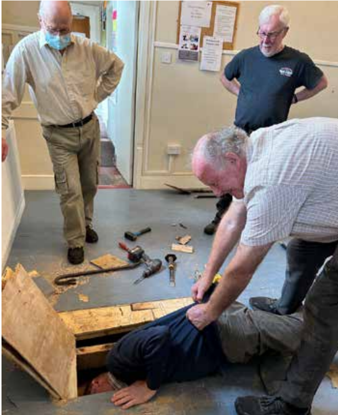
Exploring the Existing Floor Issues Brendan Howley assisted by Derry Delaney and Dan Leo
